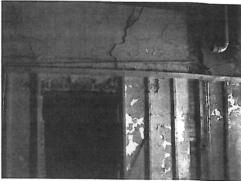
Image 4 (Crack in Common Wall )
