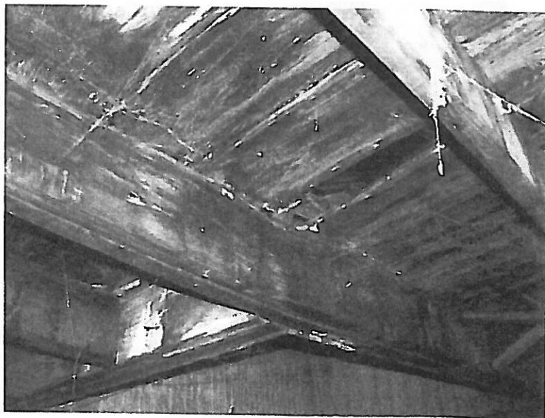
Image 7 (Skylight Roof Framing Large Deflection)
