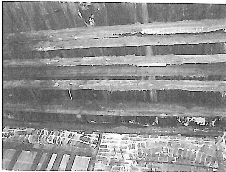
Image 9 (2x8 Roof Joists, Poor Condition)
