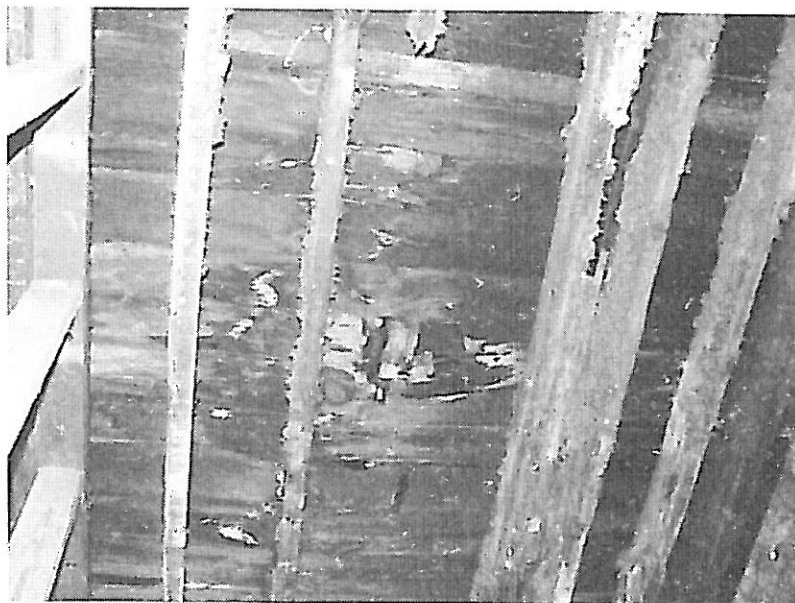
Image 11 (Roof Decking, Exposed Roof Membrane)
