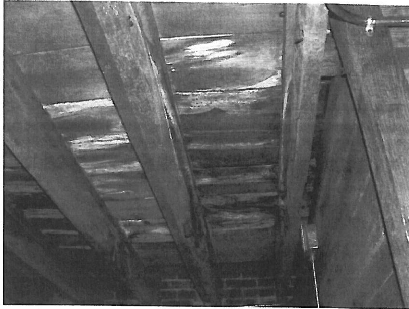
Image 12 (Water Damage, Floor Decking And Joists)
