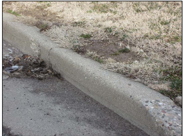
The City will use BDD funds to improve deteriorated site improvements, such as streets, curbs and gutters., sidewalks and public parking lots.
