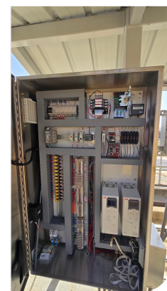
Macomb Wastewater Treatment Plant - Control Cabinet for Band Screens
