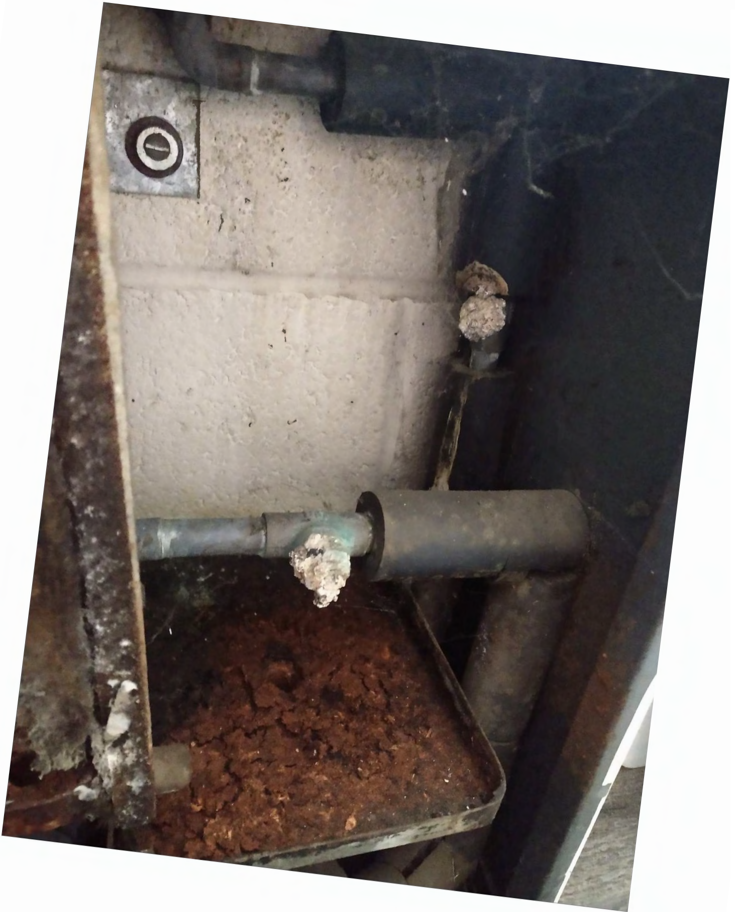
Attachment: HVAC_Pictures (2026 : Resolution No. 60-19/20 Bid Award for HVAC Improvements at the Bus Department Facility)
