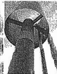
Pilot nozzles / Burner Stack
