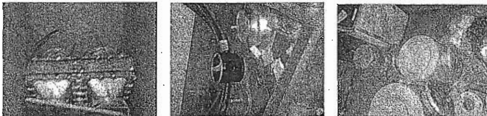
Remaining Varec Biogas equipment in warehouse storage
