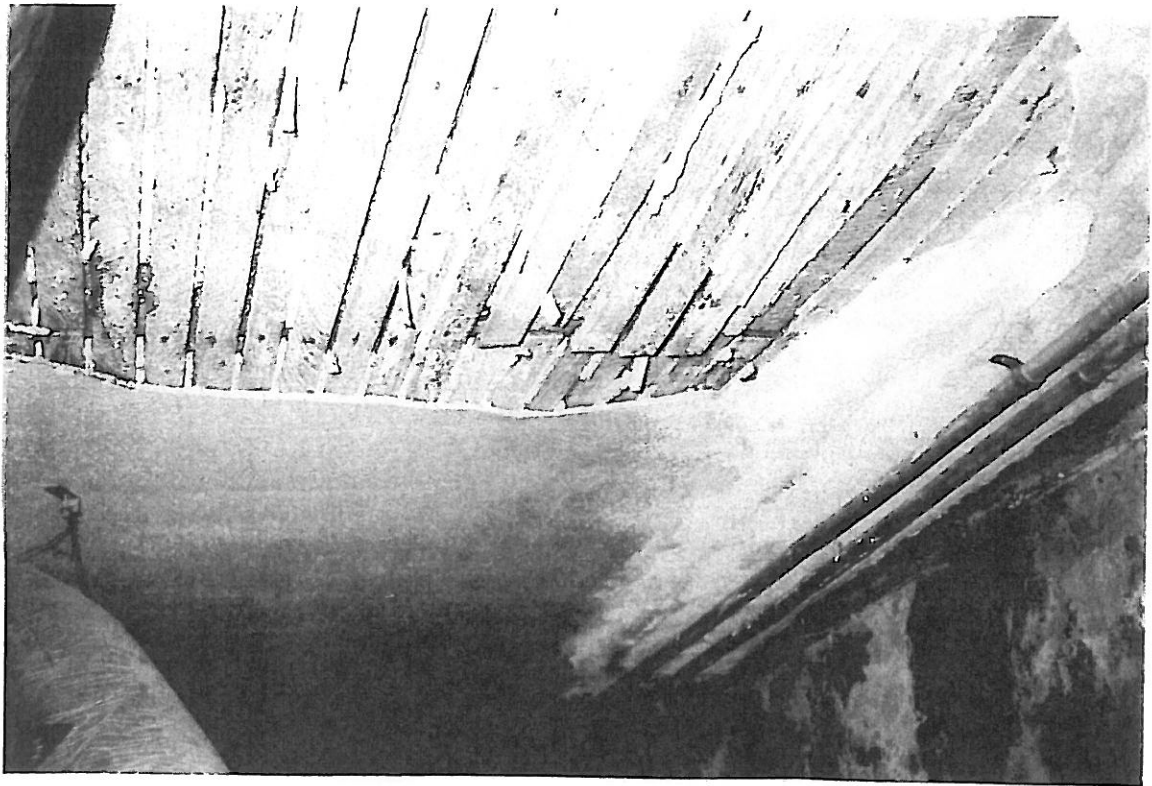
PHOTO NO. 12 - ATTIC - WATER DAMAGE TO ORIGINAL CEILING
