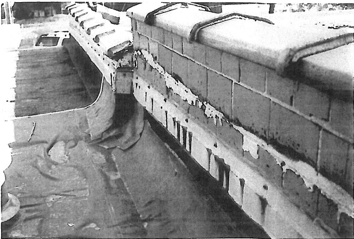
PHOTO NO. 17 - ROOF - OPEN SEAMS IN RUBBER MEMBRANE PATCH, DETERIORATED SEALANT IN METAL CAP FLASHING TROUGH, OPEN AND CRACKED MORTAR JOINTS IN CLAY TILE COPINGS, AND DETERIORATED MORTAR JOINTS IN MASONRY PARAPET
