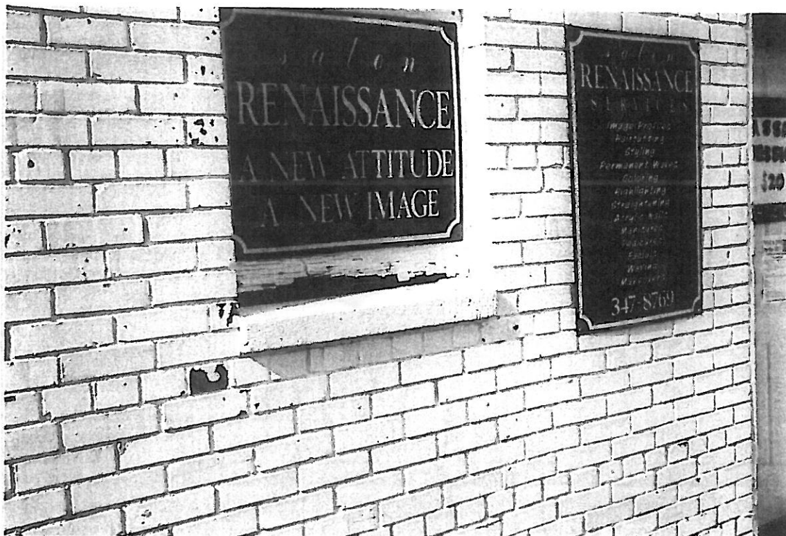
PHOTO NO. 7 - CLOSURE AT ABANDONED WINDOW
