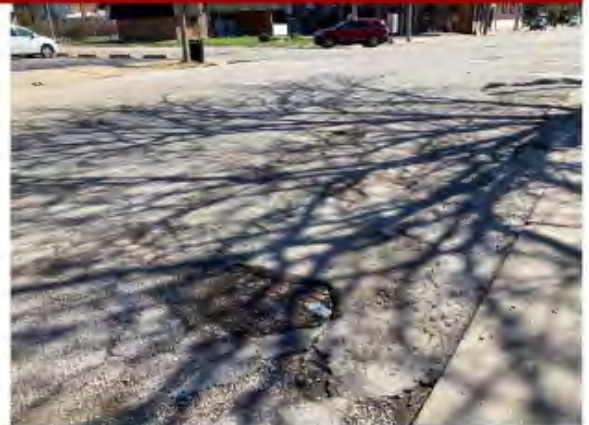
Failing overlay over original brick street
