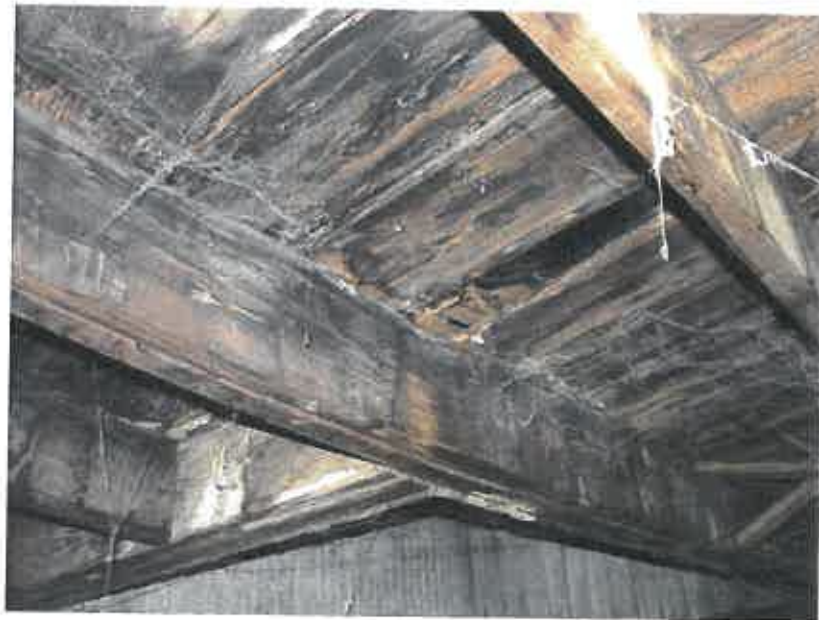
Image 7 (Skylight Roof Framing Large Deflection)
