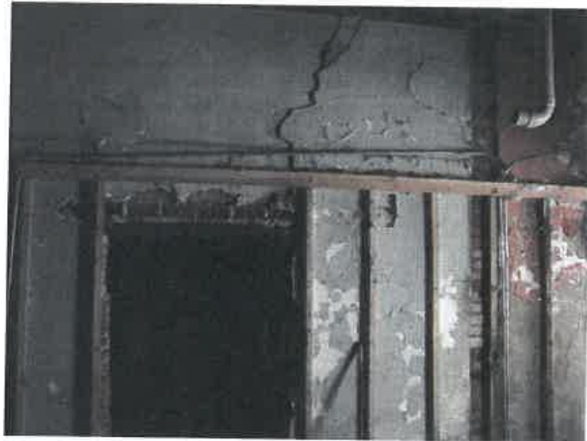
Image 4 (Crack in Common Wall )
