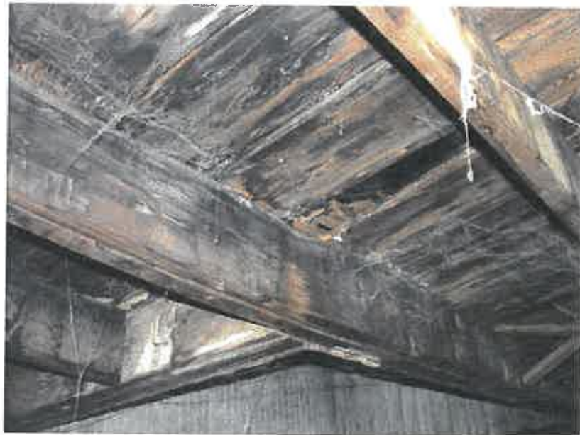
Image 7 (Skylight Roof Framing Large Deflection)
