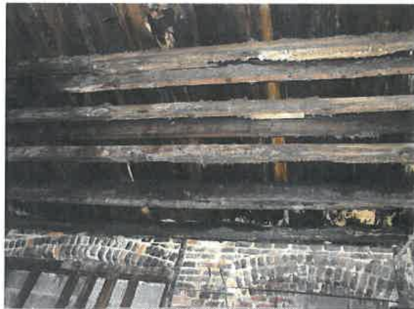
Image 9 (2x8 Roof Joists, Poor Condition)
