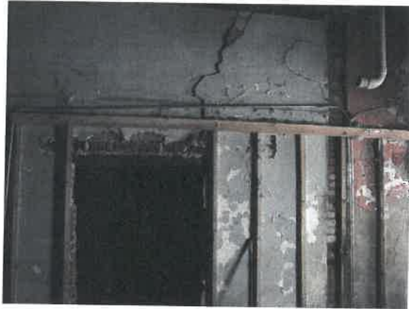
Image 4 (Crack in Common Wall )
