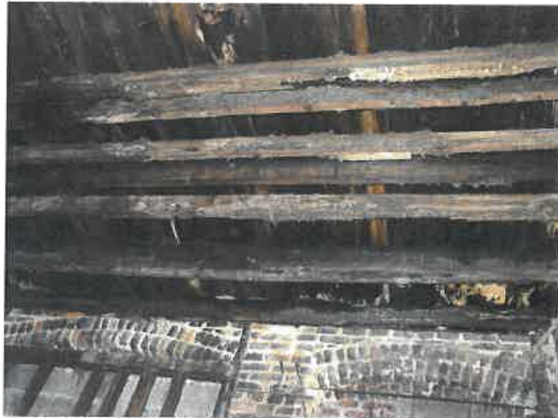
Image 9 (2x8 Roof Joists, Poor Condition)
