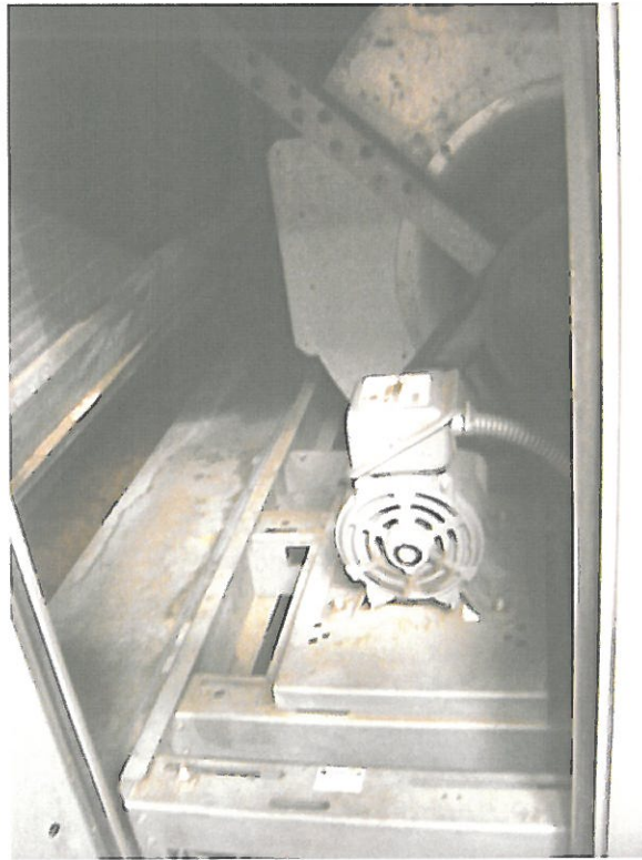
Picture 5 – AHU Supply Fan
